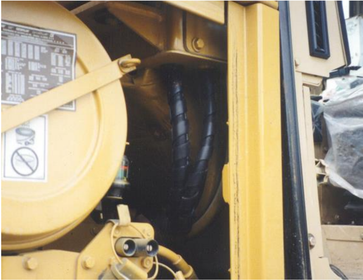
Hoses into evaporator box.
