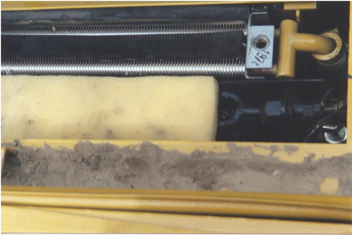
Top of evaporator assembly in heater box.
